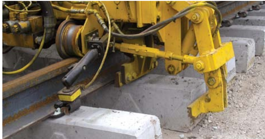
Clipping is carried out by a Nipper-Clipper mechanism on the New Track Construction Machine.
