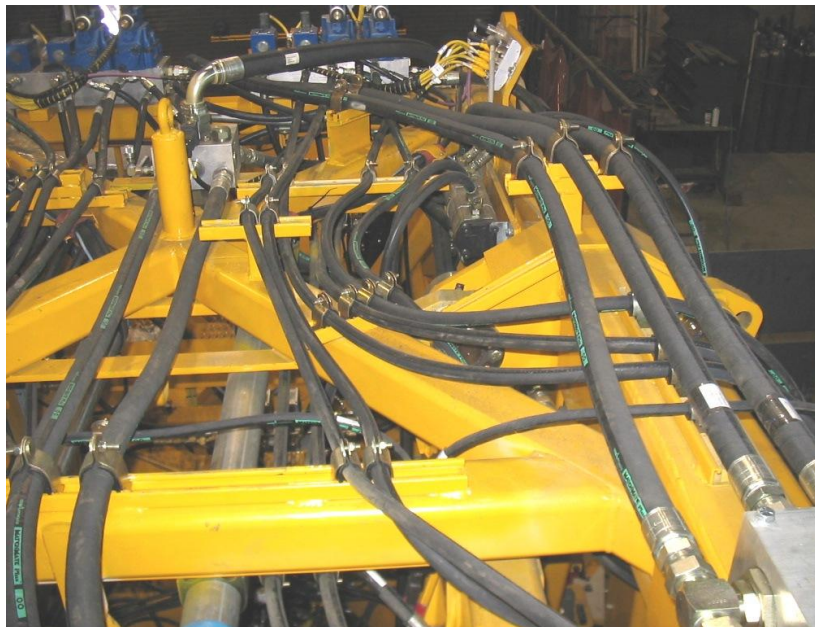
FIGURE 3 #16 HOSES BEFORE CONVERSION
